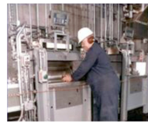
Kiln Feed Room
