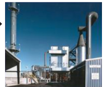
Air Pollution Control System
