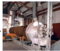
Rotary Kiln Incinerator
